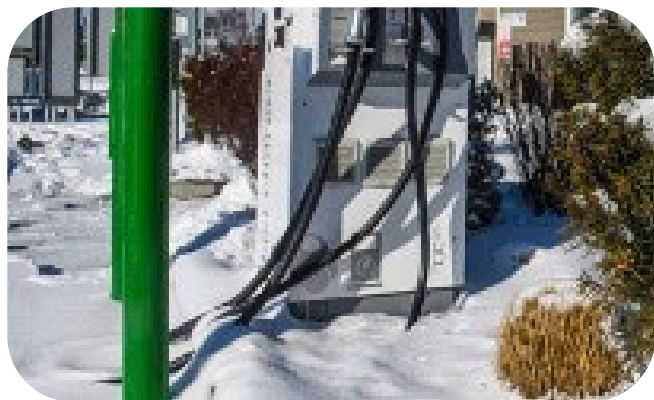
Cables buried by snow and ice
